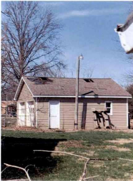
Deteriorated and Fire Damage – 720 W Hwy 50
