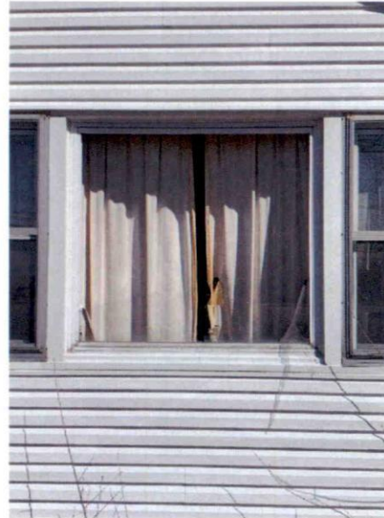
Deteriorated and Unsafe Conditions- 722 W Hwy 50
