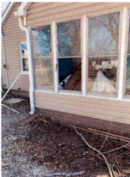
Deteriorated and Unsafe Conditions- 720 W Hwy 50
