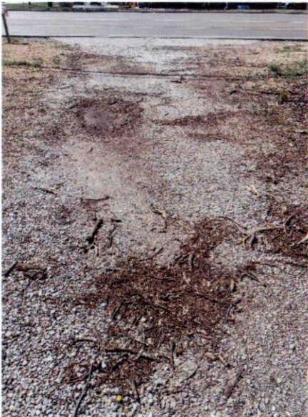
Deteriorated Driveway- 720 W Hwy 50
