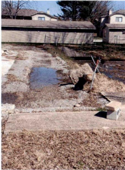
Deteriorated and Demo Materials – 1614 N Green Mount Rd
