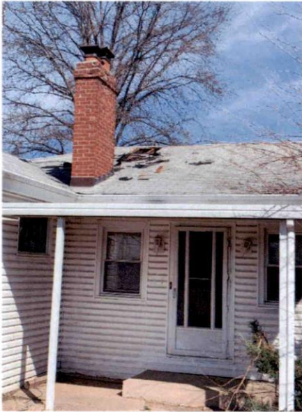
Deteriorated and Fire Damage- 722 W Hwy 50
