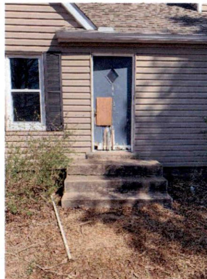
Deteriorated and Unsafe Conditions- 720 W Hwy 50
