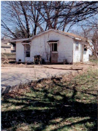
Deteriorated and Unsafe Conditions – 720 W Hwy 50
