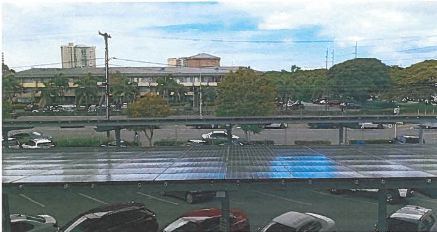
Using solar panels to generate energy and provide shading for a parking lot.
