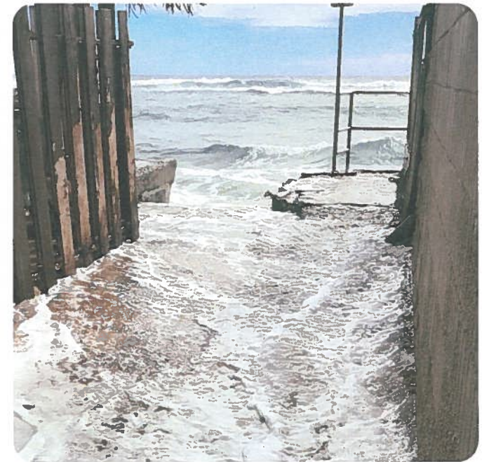
An inundated beach access walkway (Source: UH SOEST King Tides Project)
