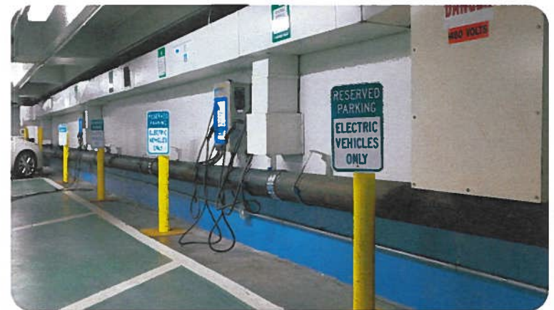
Parking facility with electric vehicle charging stations.
