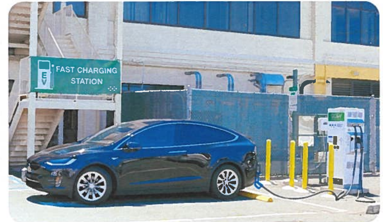
EV fast-charging station at the Hawaiian Electric lot
