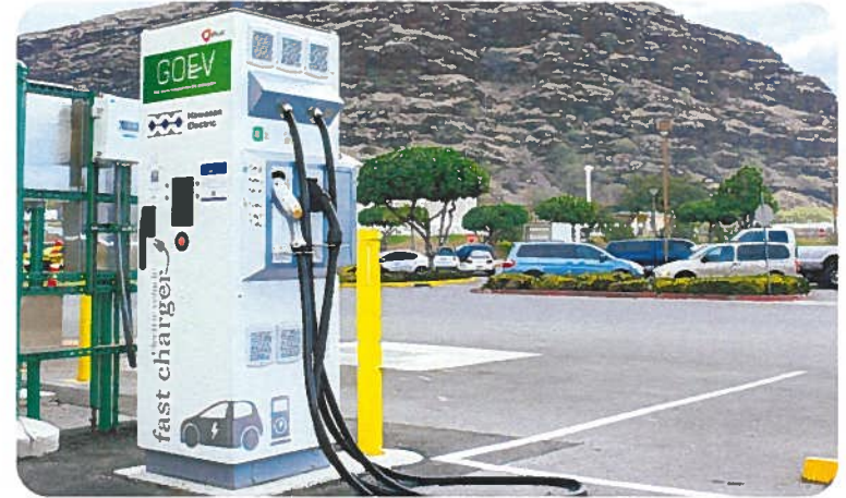
Surface parking lot with a fast charger.
